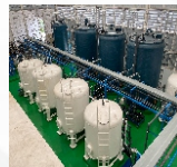
Thermal Storage / Buffer Tanks
