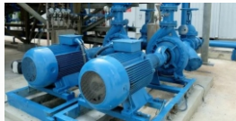
Variable Primary Pumps
